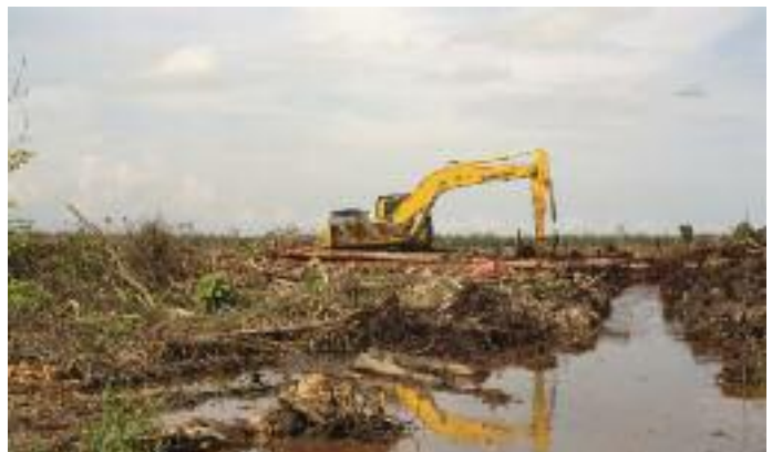
New land clearing, digging of drainage canal in Indonesia. © Jason Taylor / FoEI
